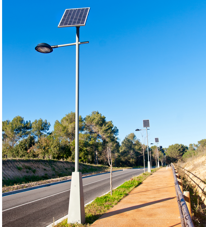
Figure 20. Solar-power street lighting system.
